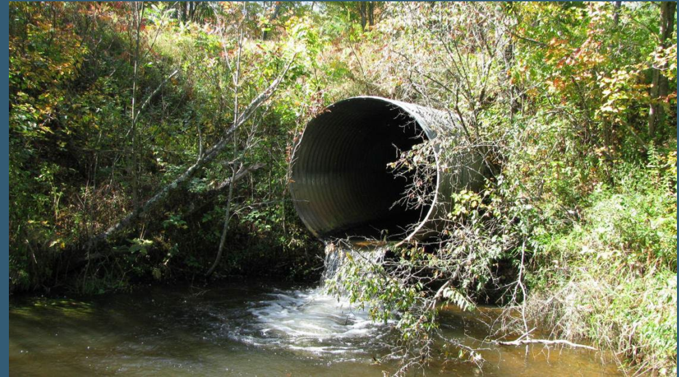
Perched culvert above streambed
