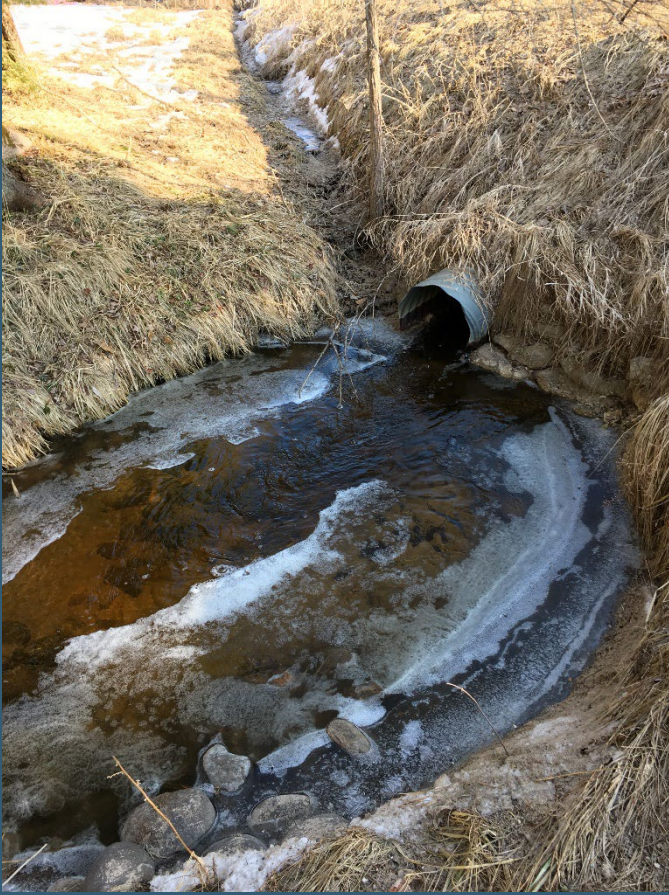
Scour hole downstream
