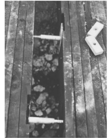
Figure 10—Connection between half-width panels was achieved by placing couplers on adjacent bars and stressing the entire deck together.
