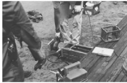
Figure 7—High strength steel bars were tensioned using a single hydraulic jack, electric pump, and steel chair.
