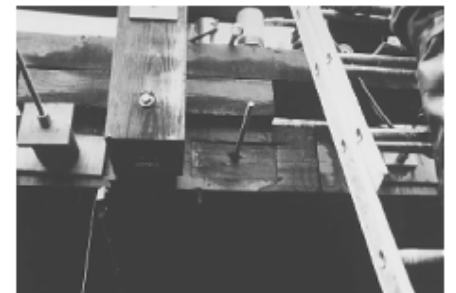
Figure 29—Visible crushing of approach span, Eastern Hemlock lumber lamination, observed after the removal of the bearing plate at the final site visit.
