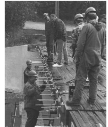
Figure 11—Two sets of deck stressing equipment were used to tension the stressing bars after deck placement.
