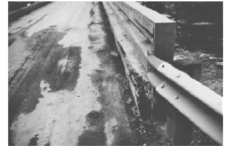
Figure 27—Vehicle damage to curb and rail system observed during a site visit near the end of the monitoring period.
