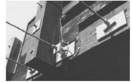
Figure 13—One of six load cells installed on stressing bars to measure changes in bar force.
