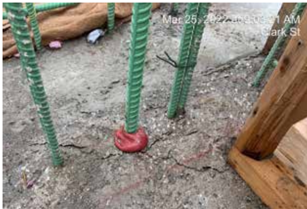
This shows the concrete around an adhesive anchored bar after the required field test was performed. The cracks in the concrete are along the failure plane.
