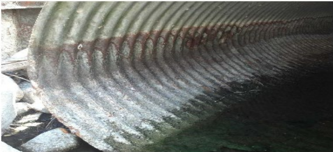
Corrosion and scale on interior of culvert
